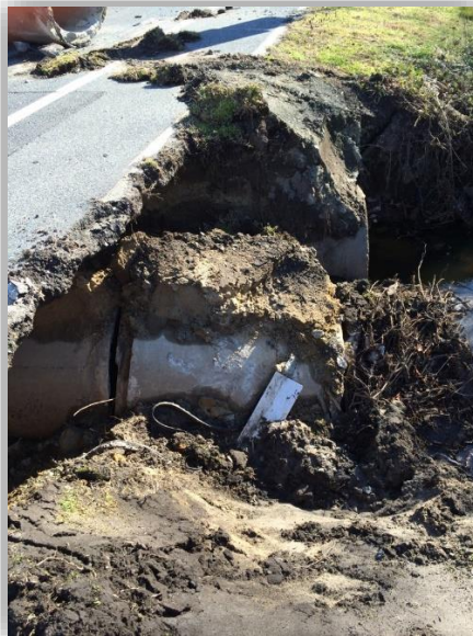
Central Avenue Pipe Failure
